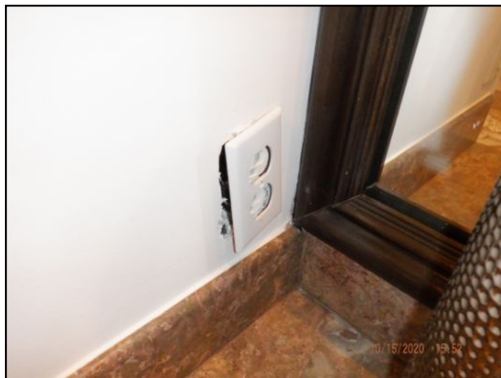
Loose outlet Master
