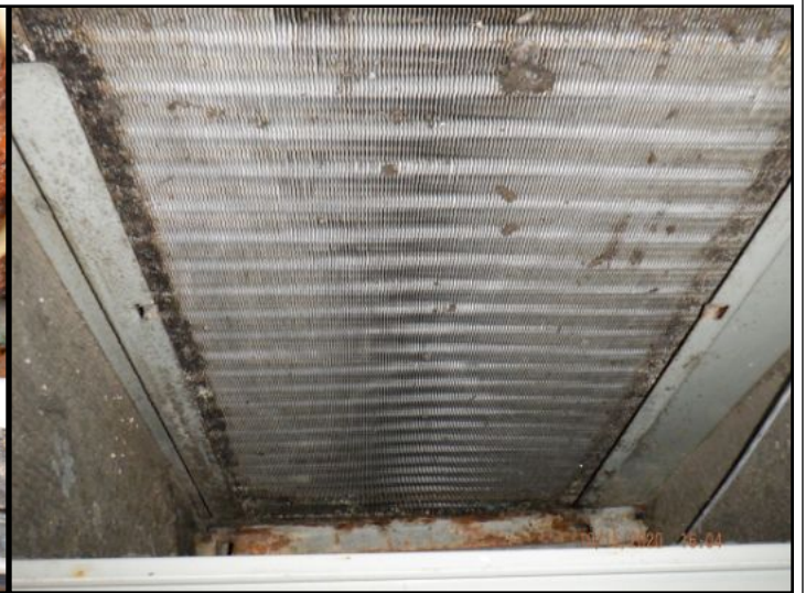
Master air handler dirty coils
