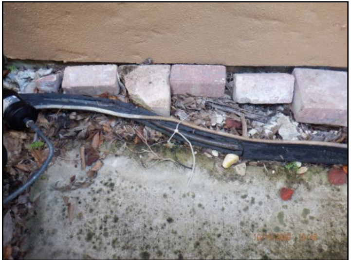
West Insulation damage
