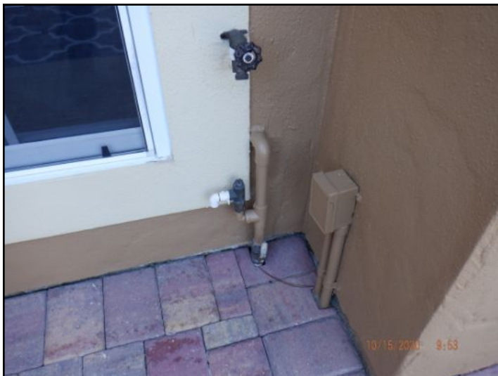
Main water shutoff location North
