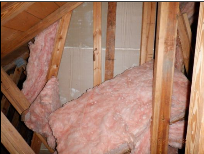
Water stains around skylight dry
