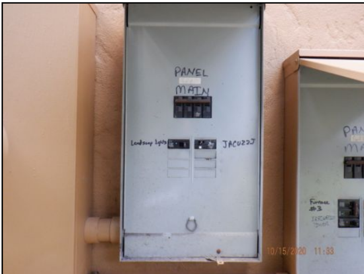
Service panel left 150 AMP
