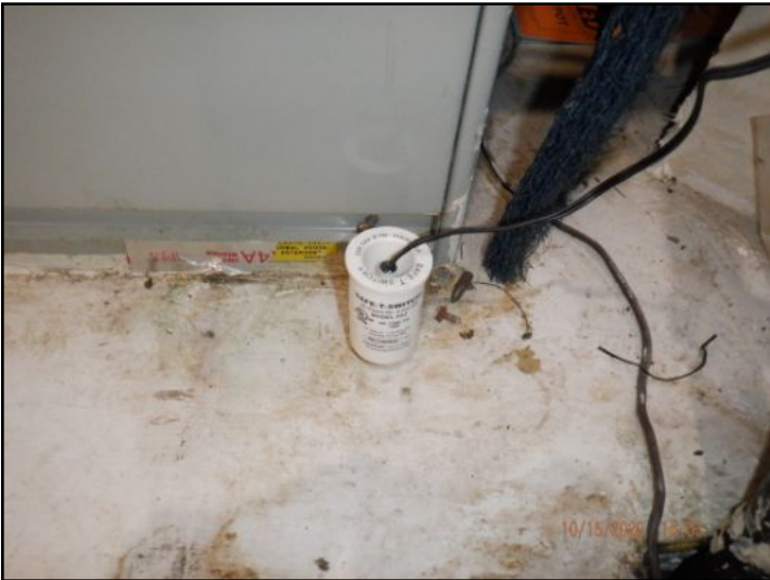
Master drain line
