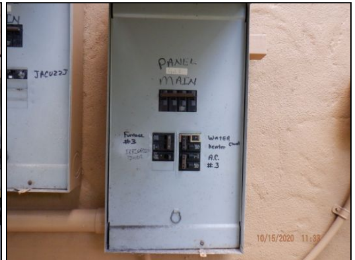
Service panel right 150AMP
