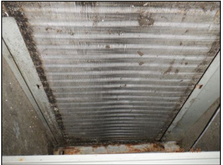
Master air handler dirty coils
