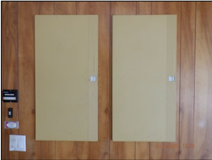
Sub panels located in garage
