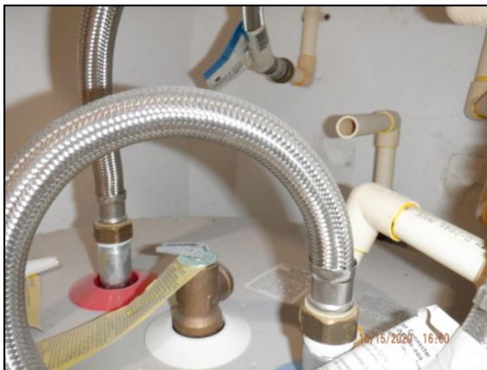
Master closet TPRV is not connected
