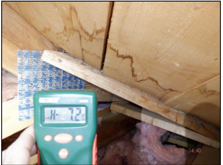
Water stains around skylight dry
