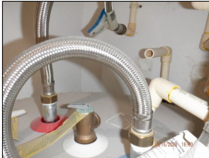
Master closet TPRV is not connected
