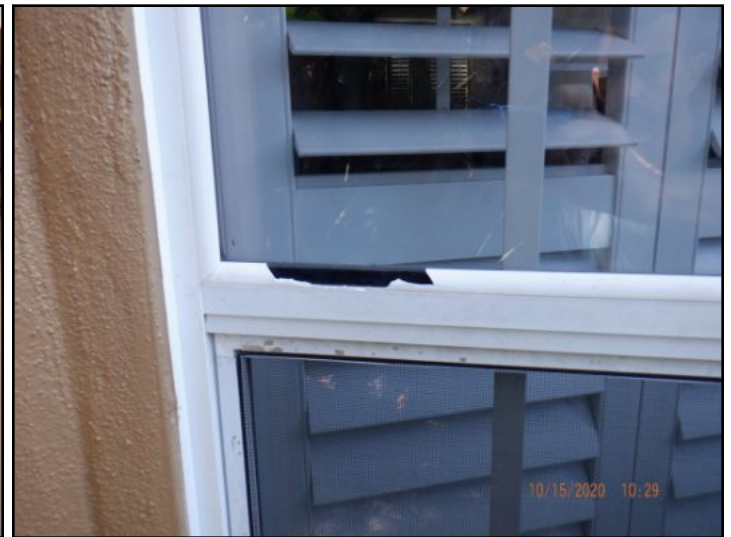
North East corner window frame damage
