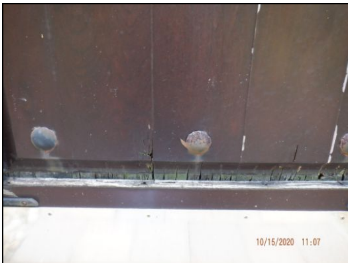
West entrance wood rot
