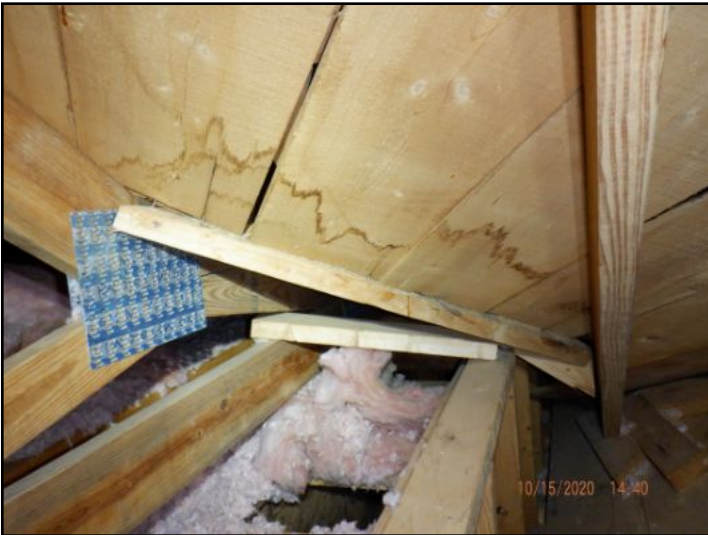
Water stains around skylight dry
