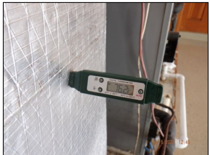
garage 76 degrees incoming
