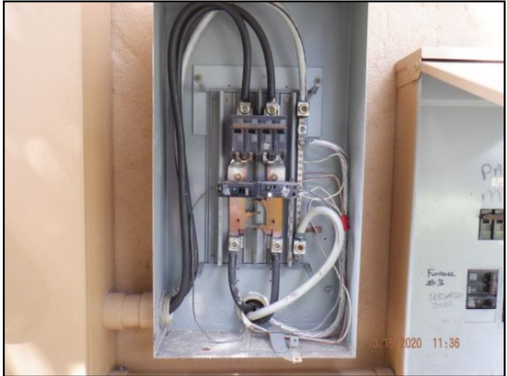
Service panel left
