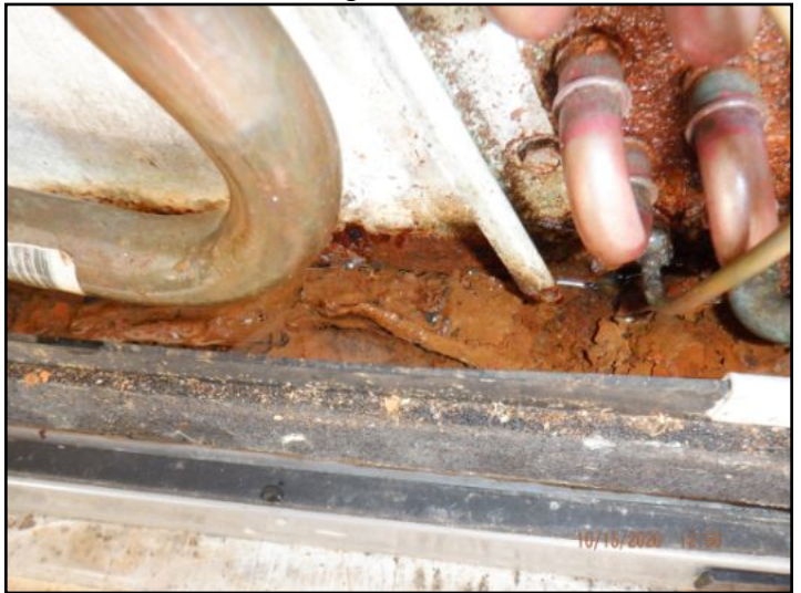
Garage air handler corrosion
