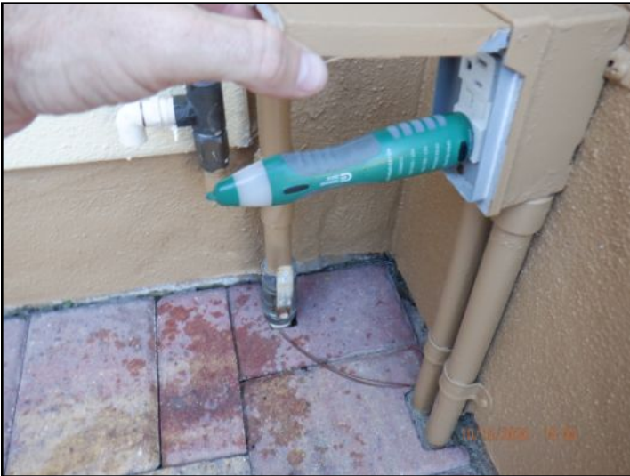
GFCI not functioning
