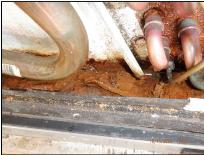
Garage air handler corrosion
