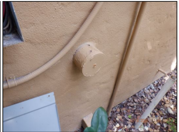
East clean out
