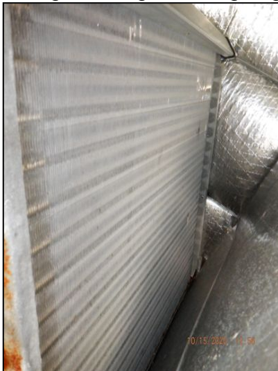
Garage air handler coils
