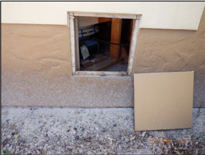
Whirlpool maintenance access NE corner exterior
