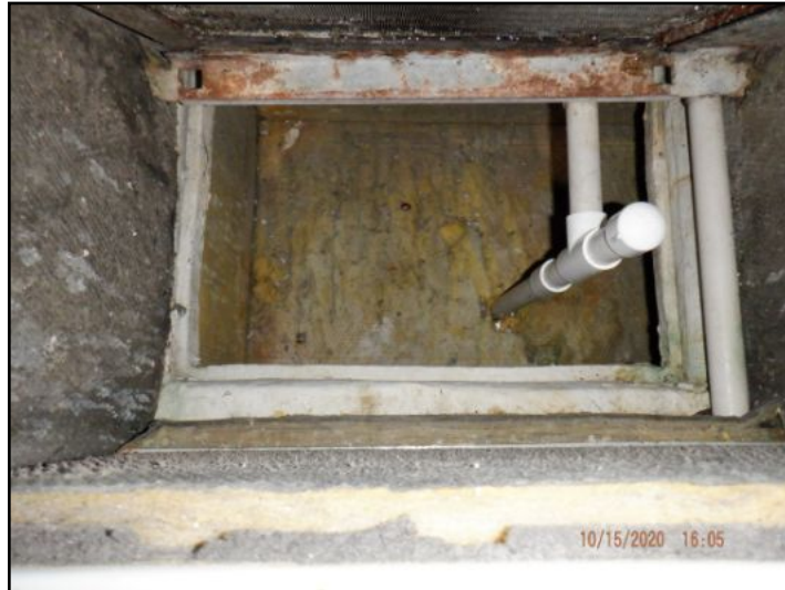
Master air handler drain line
