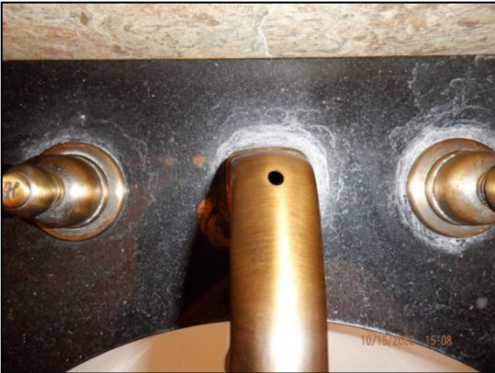
West bathroom Missing drain stopper
