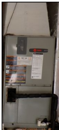
Location in garage Trane 07 3 Ton
