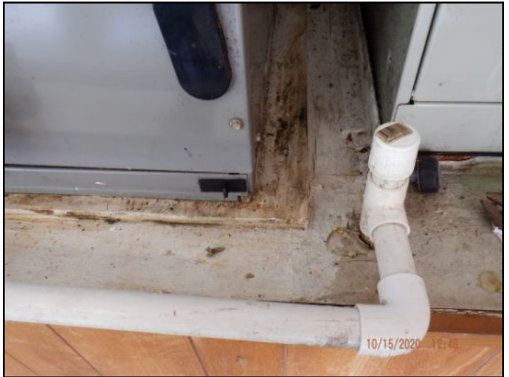
Garage drain line
