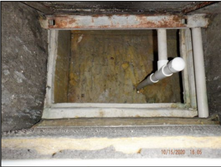
Master air handler drain line
