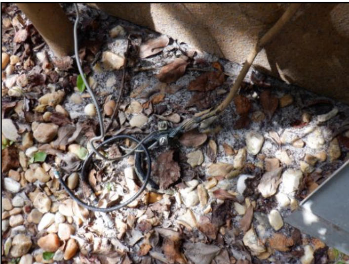
Service panel ground
