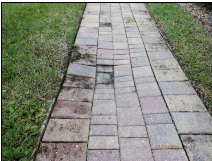
South walk way Trip hazard
