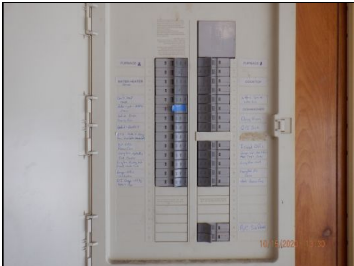
Sub panel left
