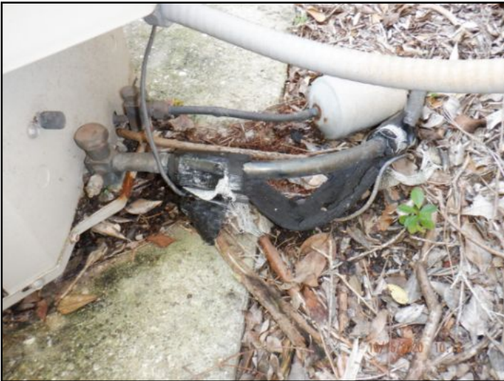
East AC Insulation damage
