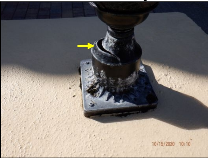
North front walkway light damage
